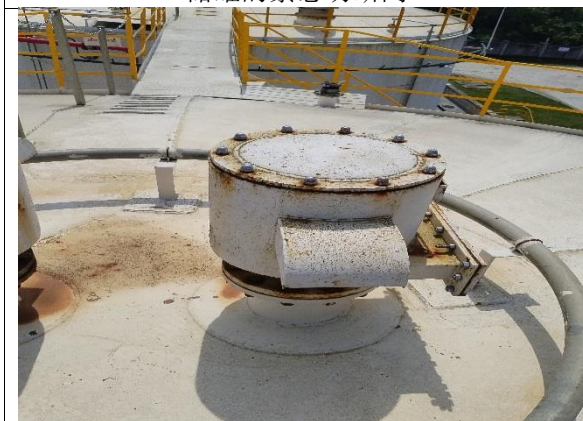
储罐的阻火呼吸阀
